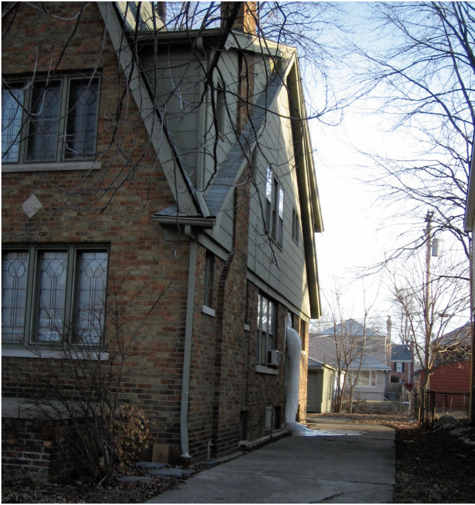
Unattended property: a frozen waterfall from a burst pipe flows out of a vacant house in Detroit that was in otherwise good condition, 2006. (Amy Hetletvedt)
