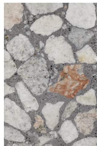
Fig. 30 The blend of the stone aggregate in the exterior curtain wall “fins” reflects the color palette of the nearby historic buildings
